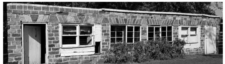
The Arnold's outbuilding reflects an art deco design in fieldstone. Note that all of the fieldstones are cut in blocks.
