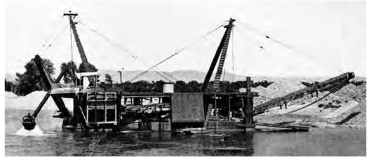
The Williams Ditch contract called for the excavation to be done with a Marion Vertical Spud Dredging Machine. Rep Photo.
